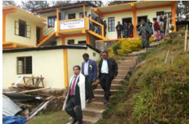
Extension of school building, repairing of Basketball court and beautification of Children's park at Mawlai Kynton Massar SSA LP & UP School, Shillong
