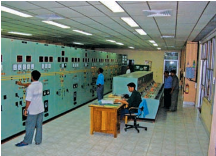
Inside view of Doyang HE plant
