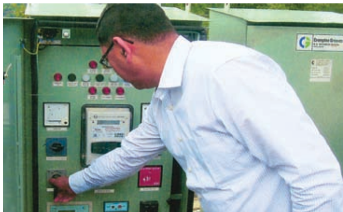
D (T) inaugurating the sub-station of Pare HE Project
