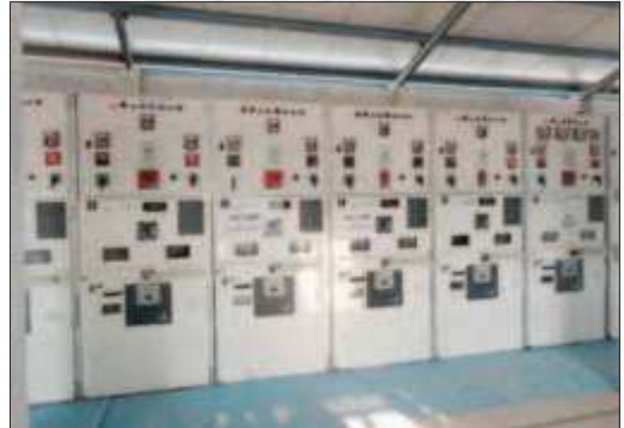
Solar Power Project, Monarchak
