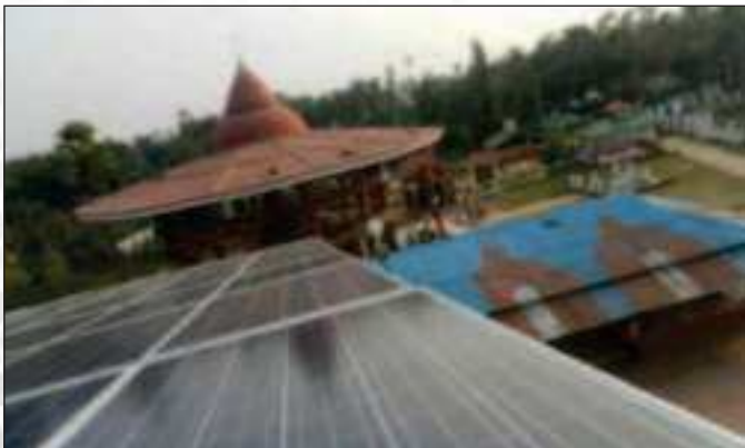
20 KW Solar panel at Khayerpur, Tripura
