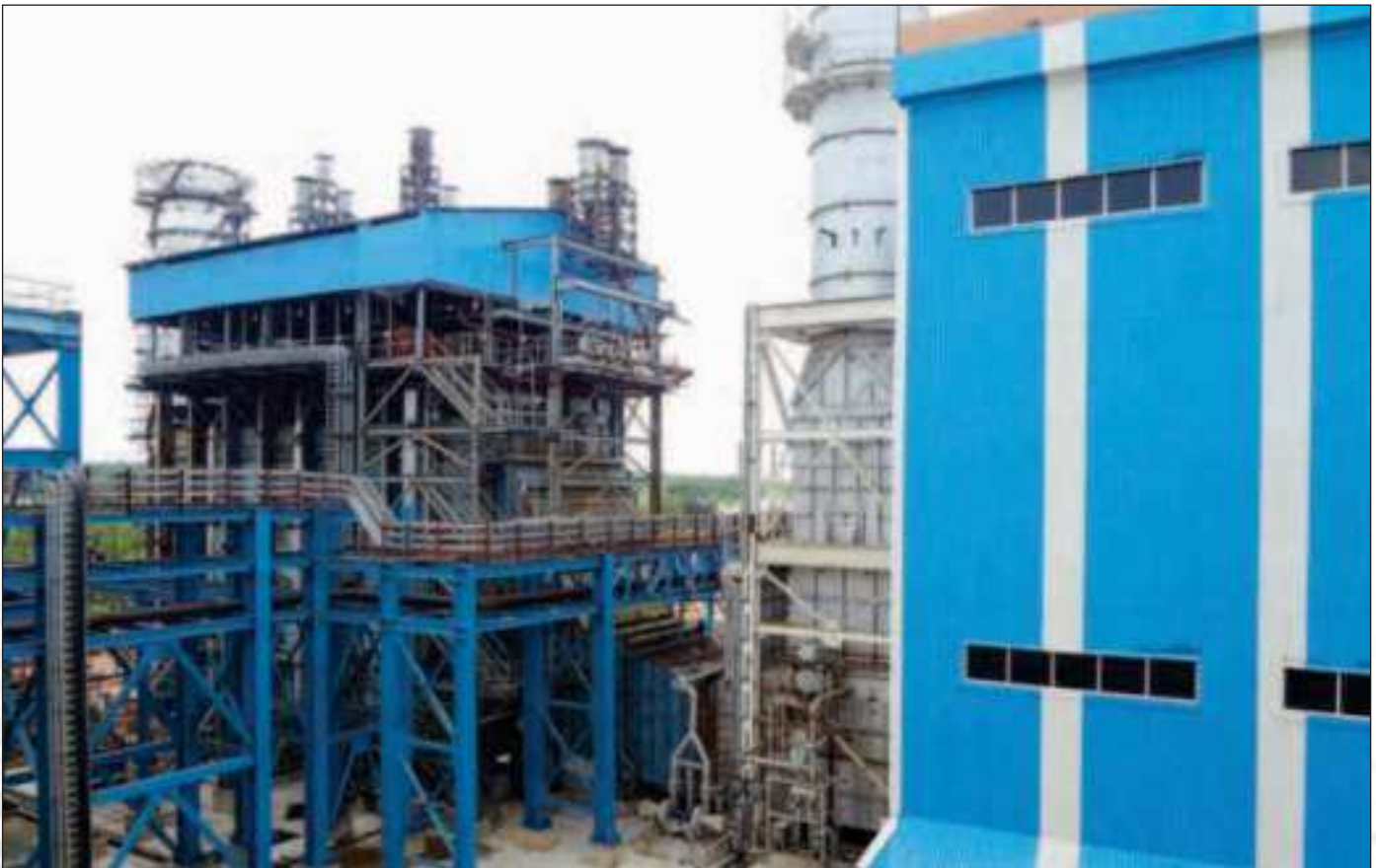
Tripura Gas Based Power Project
