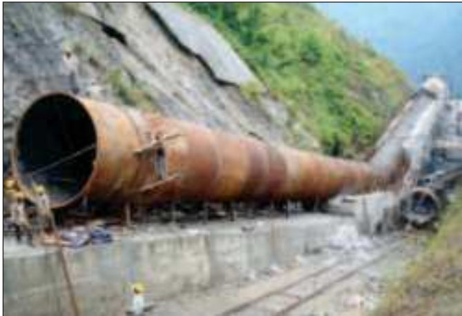
Penstock, Kameng Hydro Electric Project
