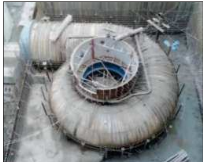
Spiral Casing Unit-I, Pare Hydro Electric Project
