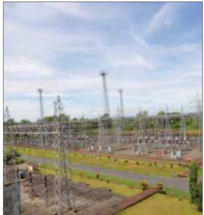
Agartala Gas Tubine Plant
