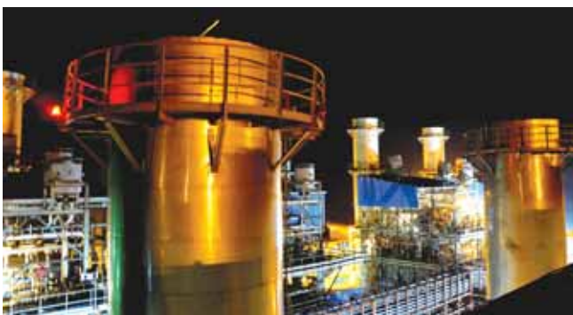
Agartala Gas Turbine Plant
