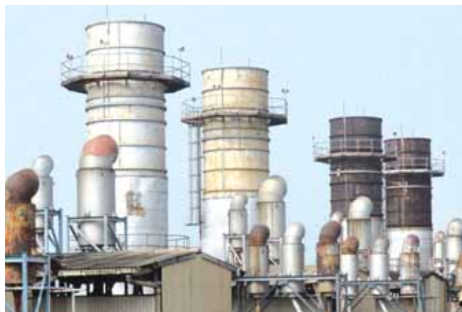
Assam Gas Based Power Plant
