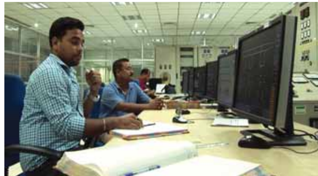
Control Room, Tripura Gas Based CC Power Project
