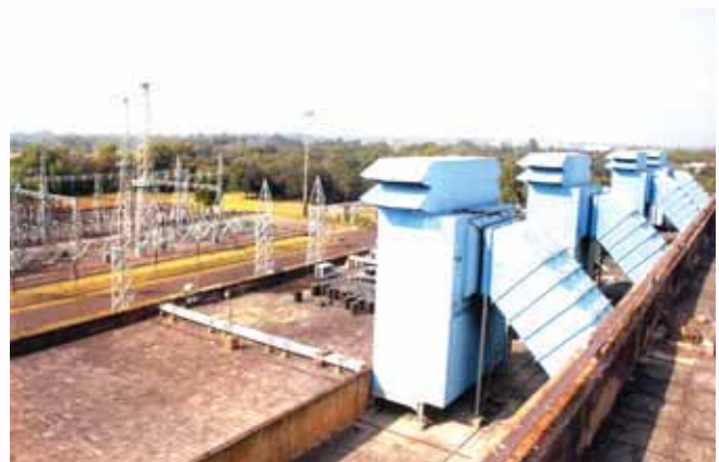
Assam Gas Turbine Plant
