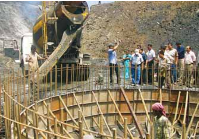
Collarring beam concreting at the vertical shaft 2 under HPT, KPC, Kameng in progress
