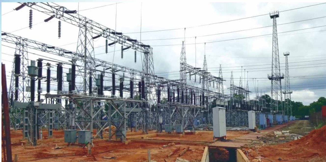
Agtrala Gas Turbine Project - Combined Cycle Extension Project switchyard
