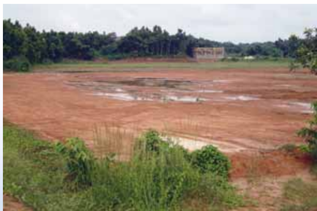
Solar Array area ready for piling at Tripura Gas Based Power Project
