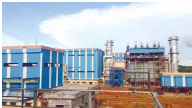
A view of Tripura Gas Based Power Project
