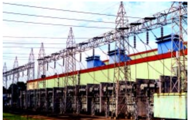
Agartala Gas Turbine Power Station
