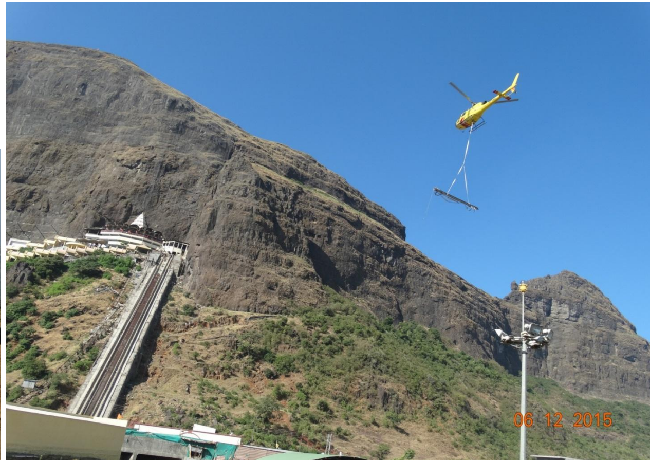
Helicopter transferring the barrier components to the temporary storage location near to the slope
