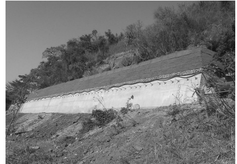
Reaction wall to prevent rockfall
