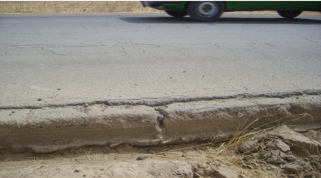
A Section of the Maiduguri-Dikwa-Gamboru Road in Borno State, Nigeria which was stabilized with Base-Seal in 2001. The shoulder was not stabilized and as a result was washed away.
