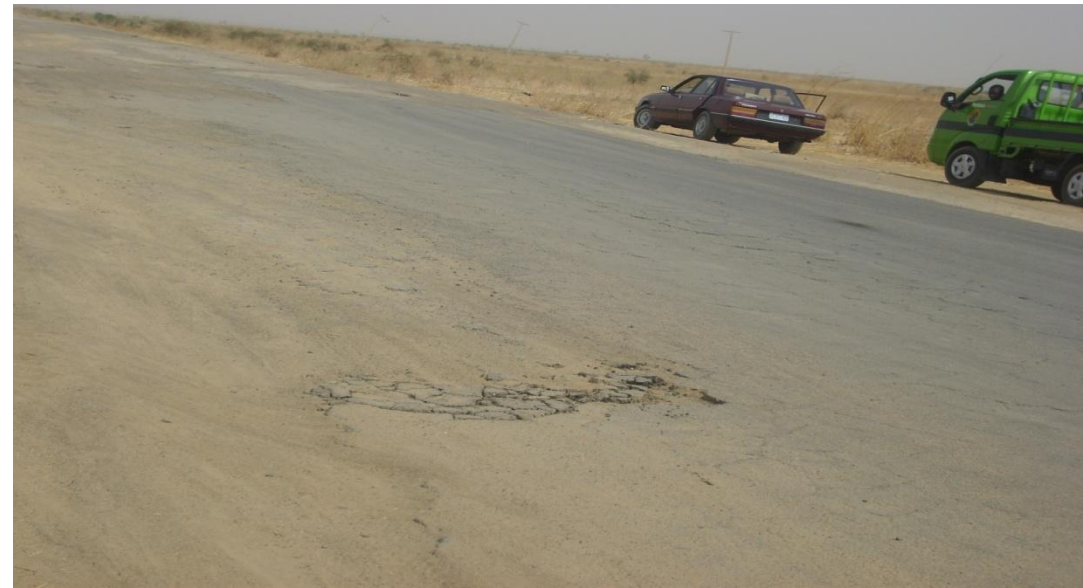
A Section NOT stabilized
