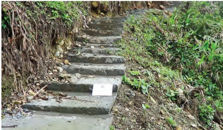
Construction of porter track with CC foot step from Khuppi 3 km to Bich Camp
