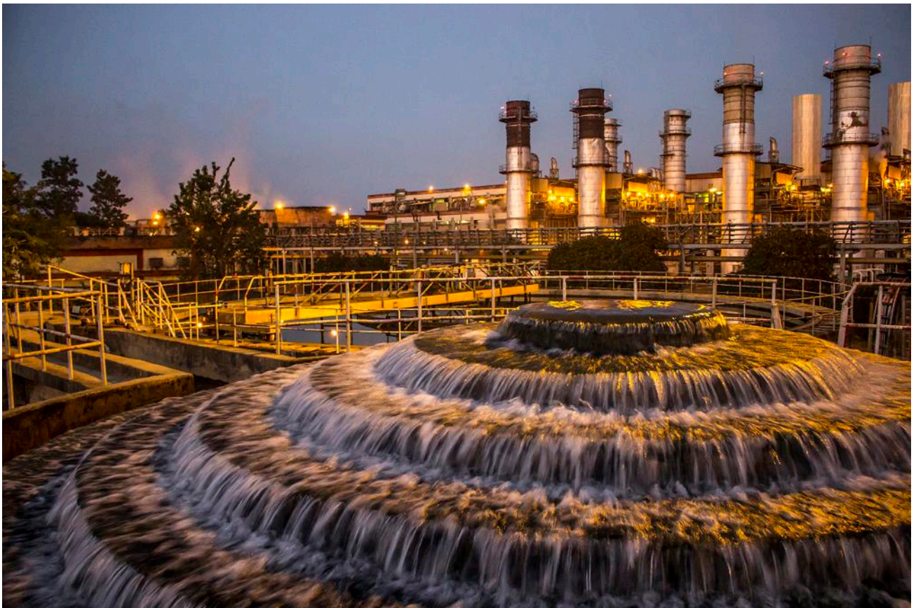
Night View of Aerator and Main Stack
