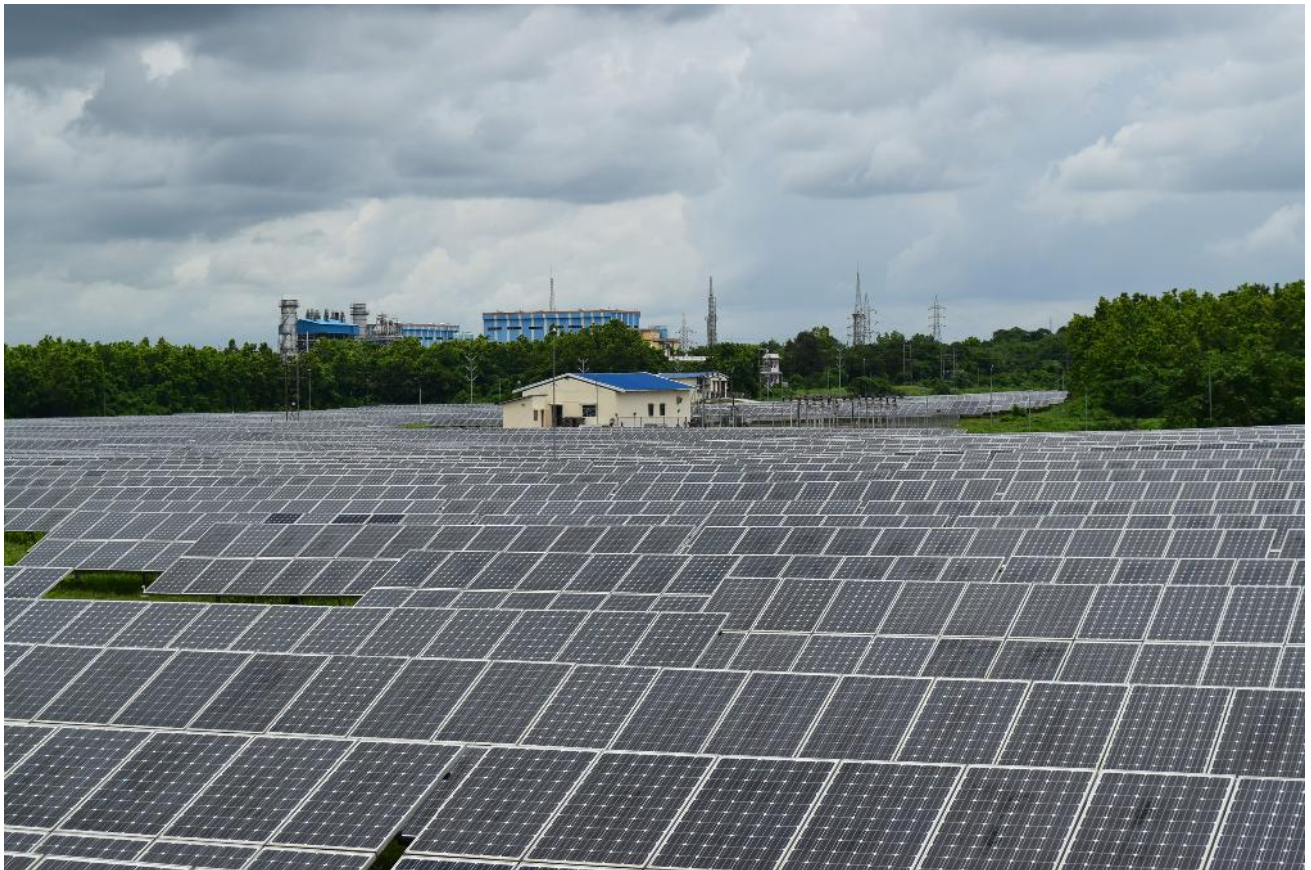
Tripura - Solar Array Area
