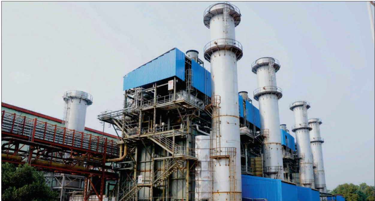
Agartala Gas Turbine Plant - Combined Cycle Extension Project
