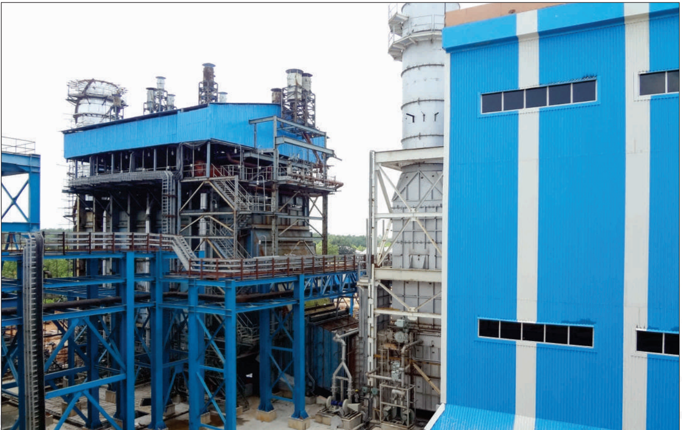
Tripura Gas Based Power Project
