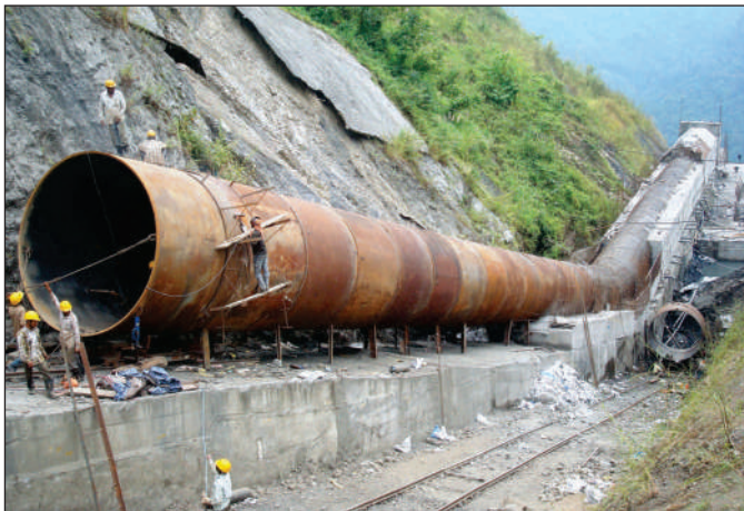
Penstock, Kameng Hydro Electric Project
