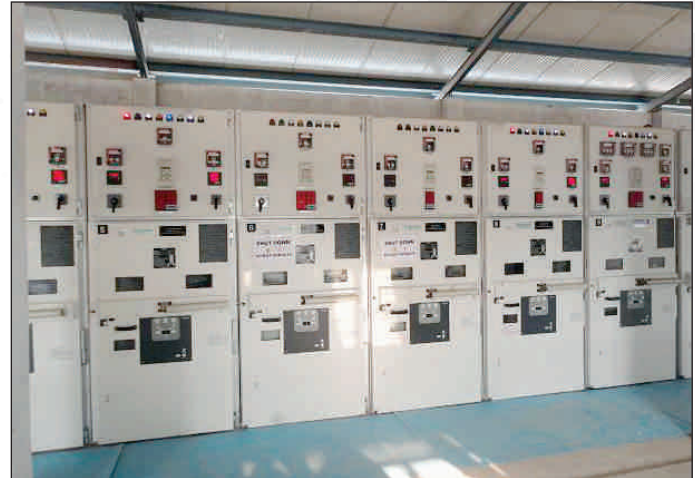
Solar Power Project, Monarchak
