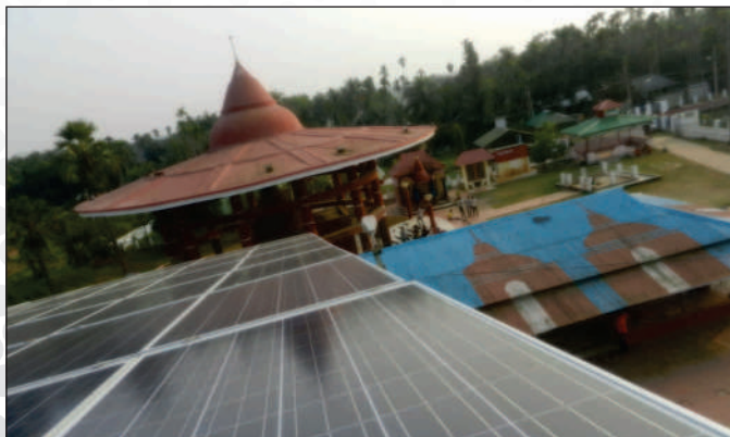
20 KW Solar panel at Khayerpur, Tripura
