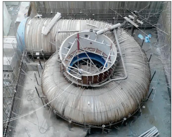
Spiral Casing Unit-I, Pare Hydro Electric Project
