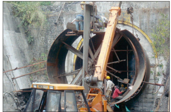
Wye-1, Kameng Hydro Electric Project
