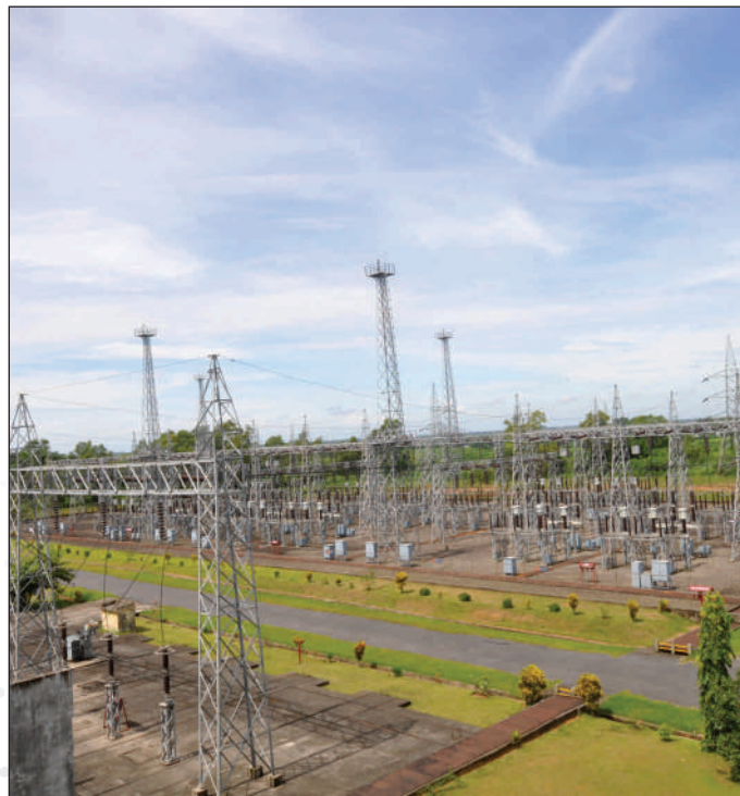
Agartala Gas Tubine Plant
