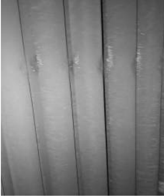
WHRS economiser tubes - dust on the fins
