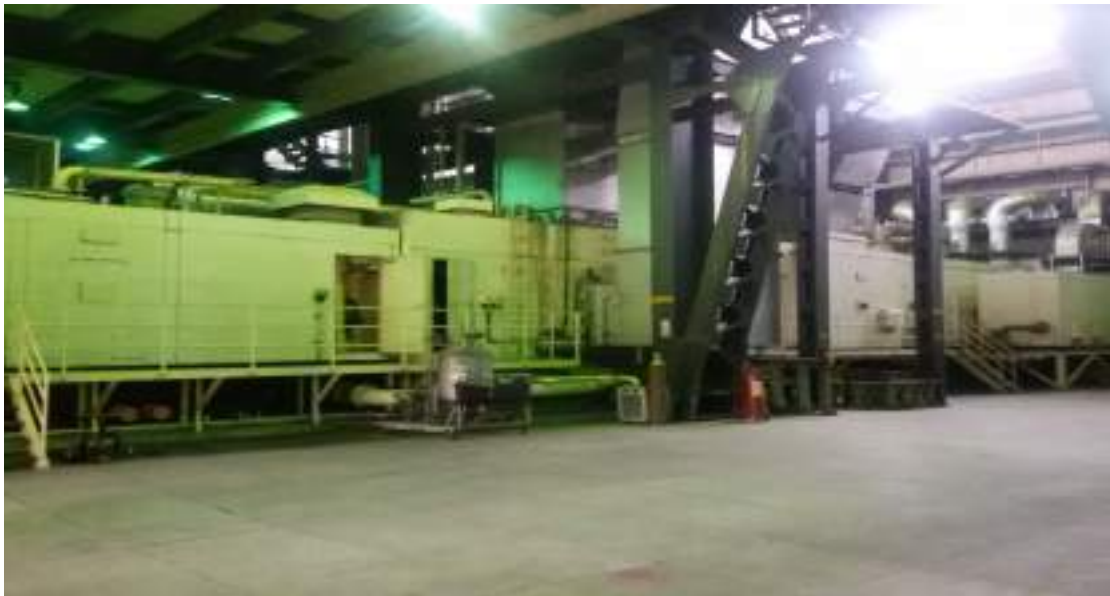
MHI Gas Turbine U#3
