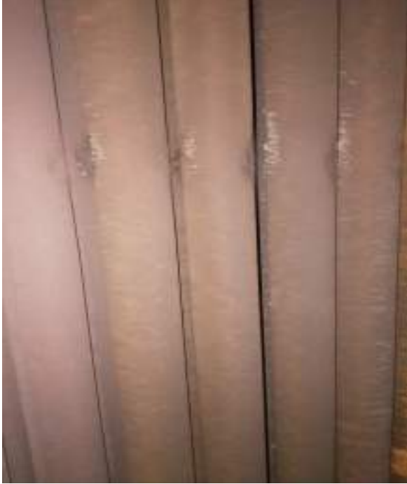
WHRS economiser tubes - dust on the fins
