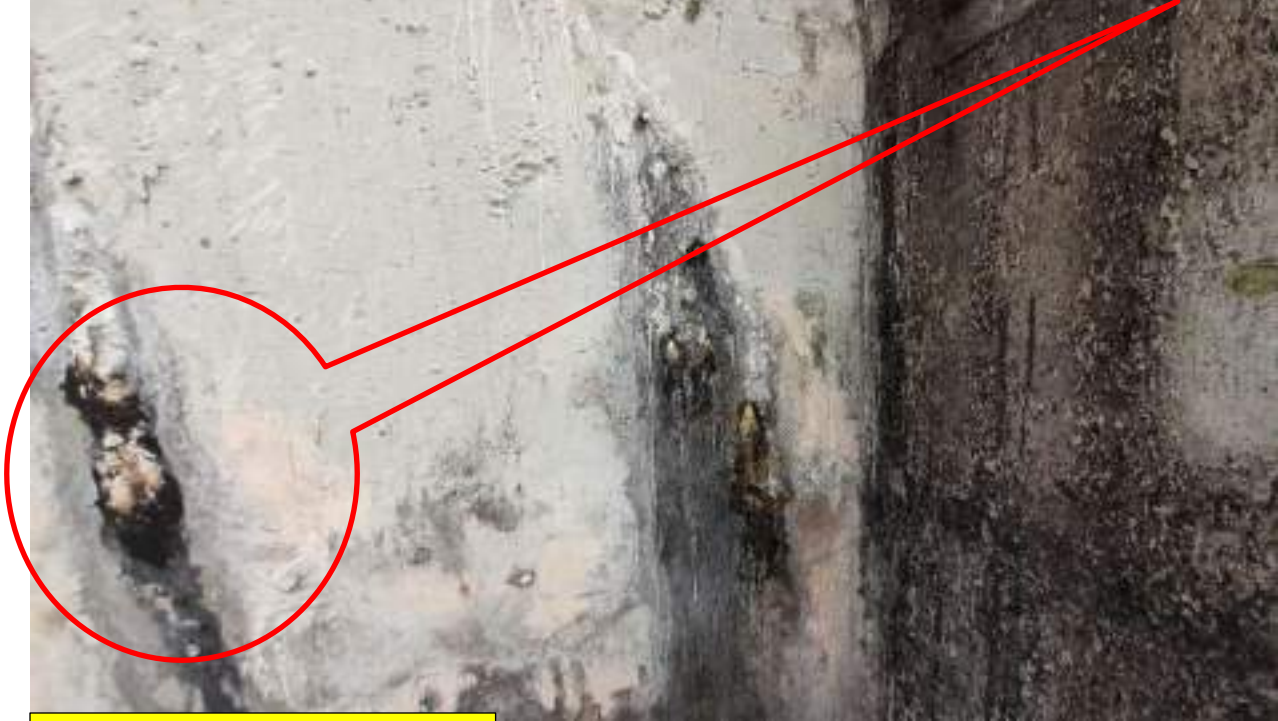
Water Leakage at wall column junction point due to severe hydrostatic pressure
