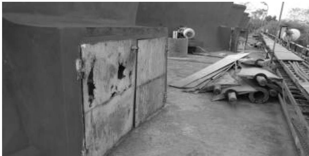
Cooling tower doors damaged
