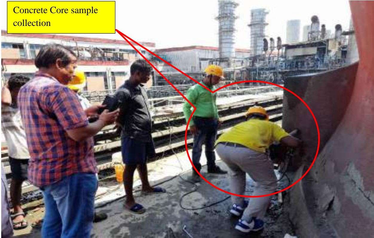
Concrete Carbonated area
