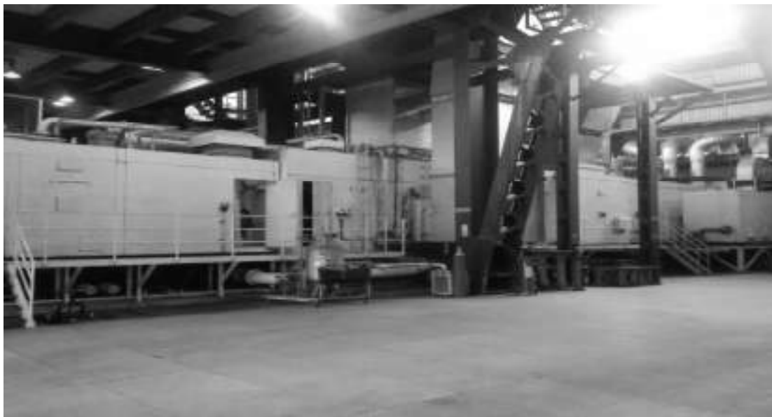
MHI Gas Turbine U#3
