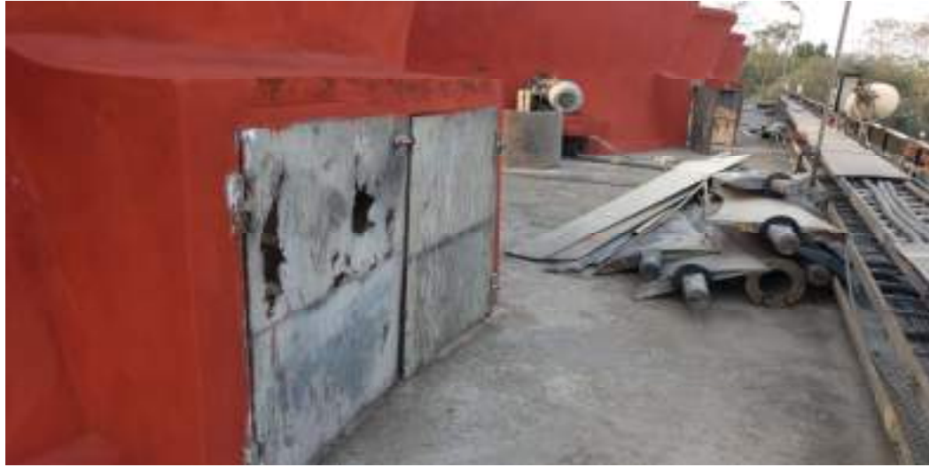
Cooling tower doors damaged
